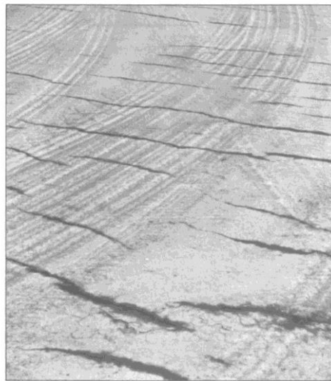
Figure 16 : Plastic shrinkage cracks in a concrete road
